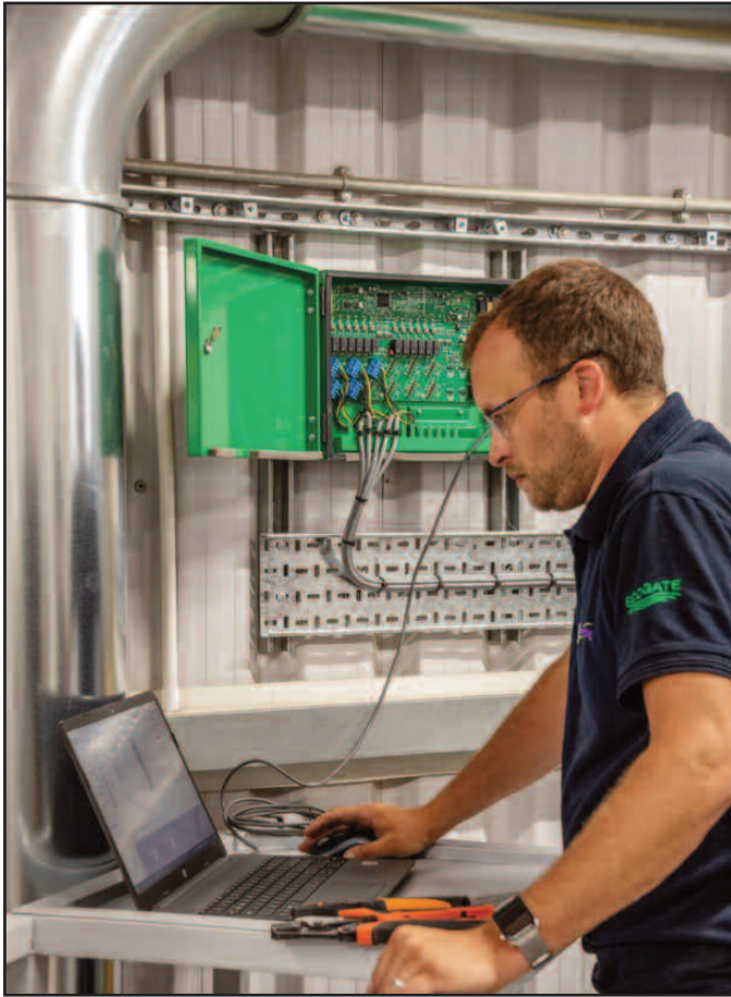
Ecogate system maintenance.
