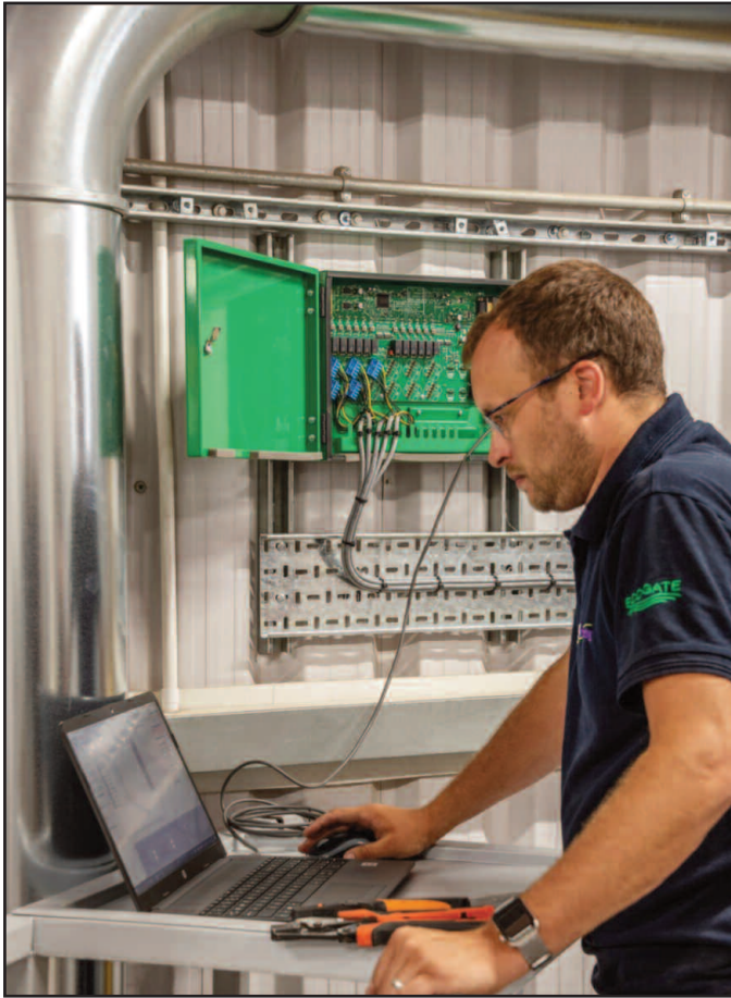
Ecogate system maintenance.
