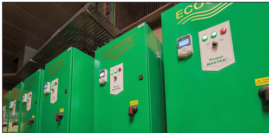
Extractly installed a total of nine PowerMASTER™ VSD units at JTC — each unit delivers precise control over the power consumed by each individual fan.
