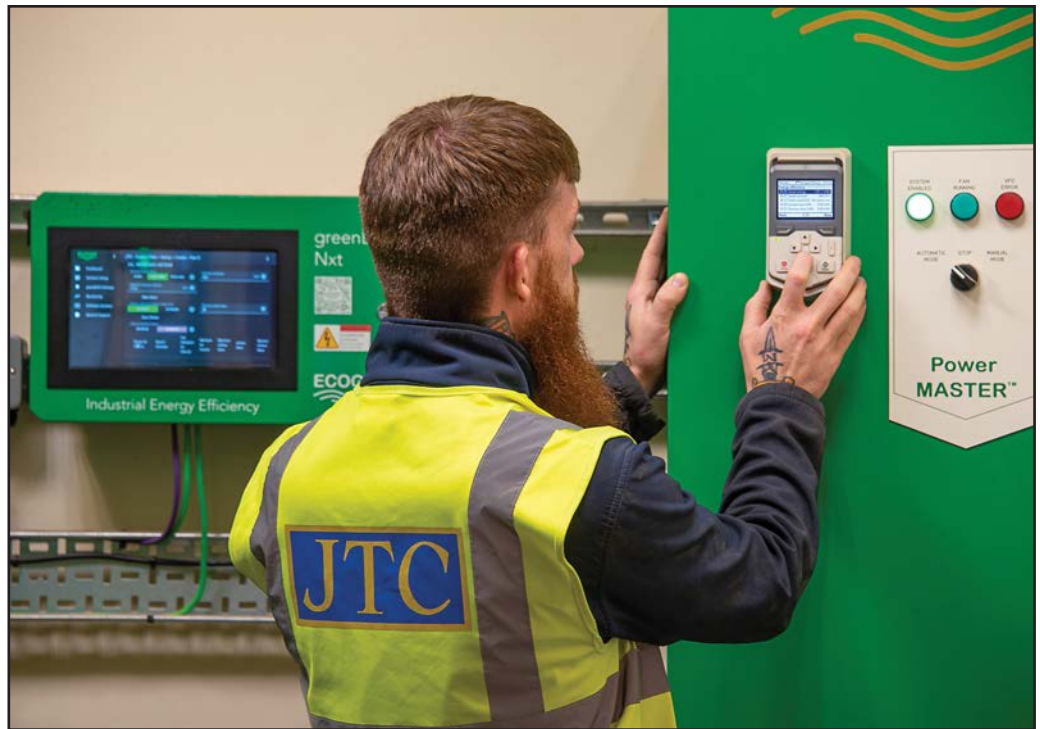
David Verrall checking stats and energy savings made to date at one of the PowerMASTER™ VSD units installed by Extractly Ltd.
