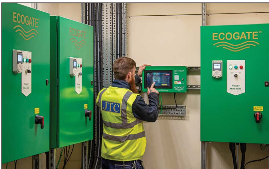
David Verrall interrogating system performance data at one of the greenBOX® Nxt units that monitors extraction demand and determines optimum speed for three of the main fans.
