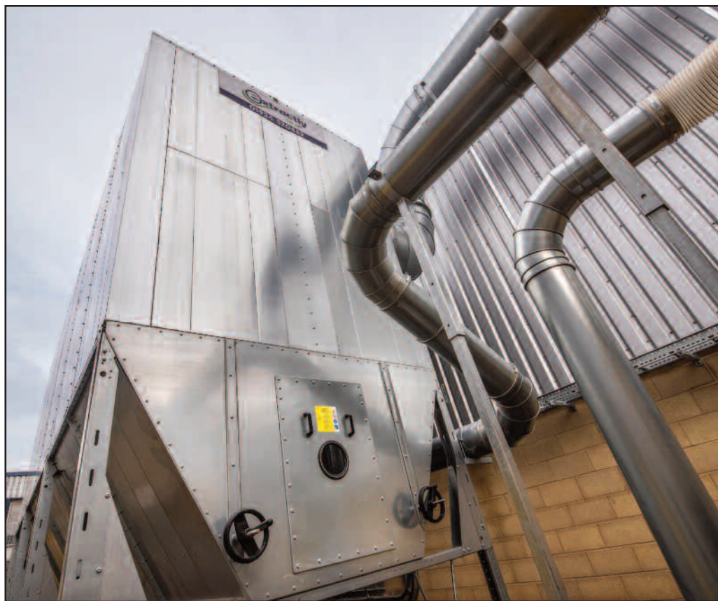
The six-module Nederman NFKZ3000 unit supplied and installed by Extractly Ltd.
