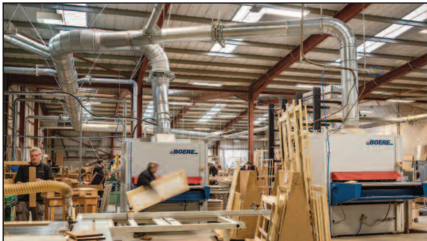
The two Boere sanders naturally require high-powered extraction when running but, with Ecogate® installed, energy consumption is significantly reduced when the machines are idle.
