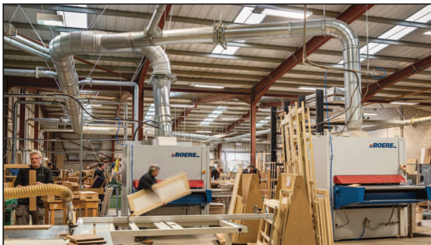
The two Boere sanders naturally require high-powered extraction when running but, with Ecogate® installed, energy consumption is significantly reduced when the machines are idle.
