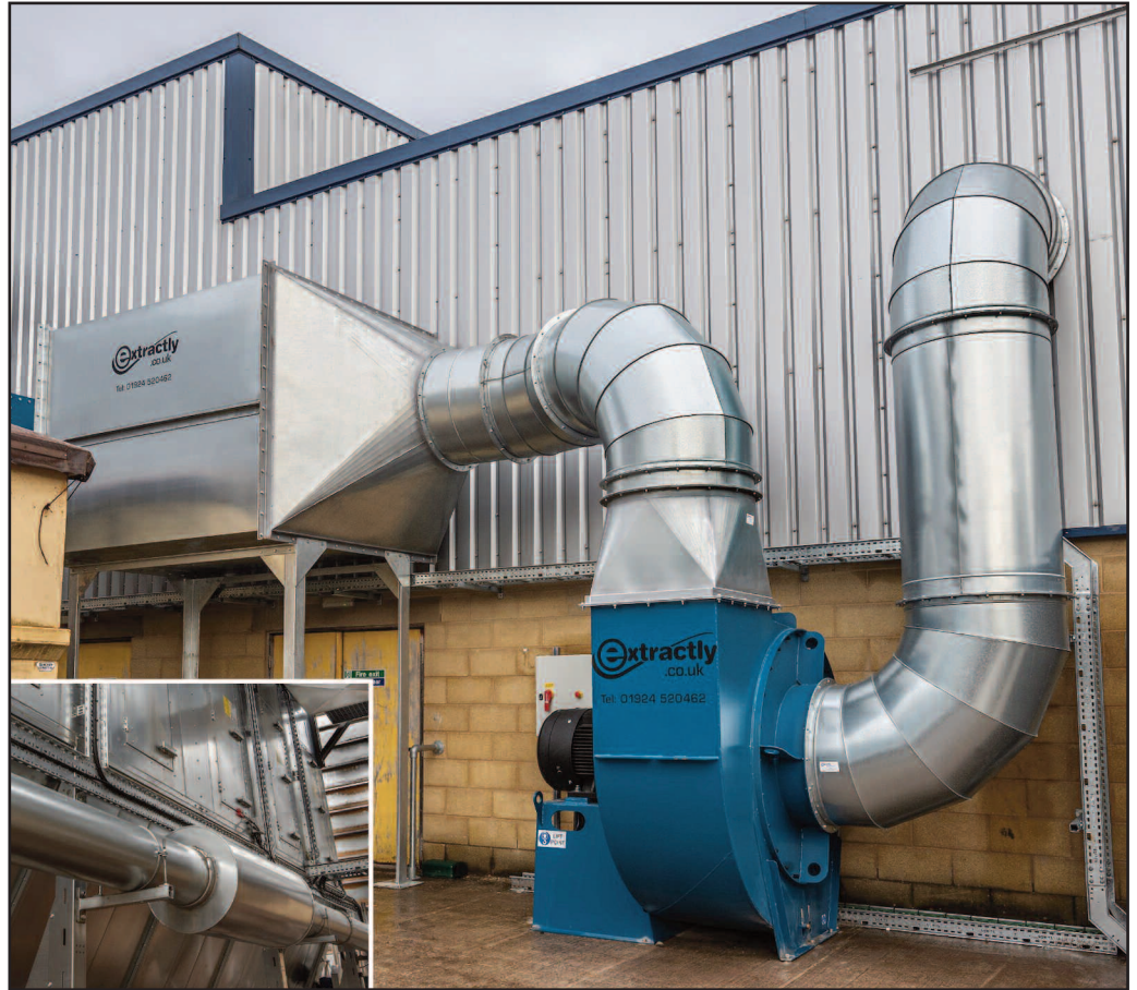
Bespoke absorptive silencers significantly reduce noise levels from the 90 kW main fan.
