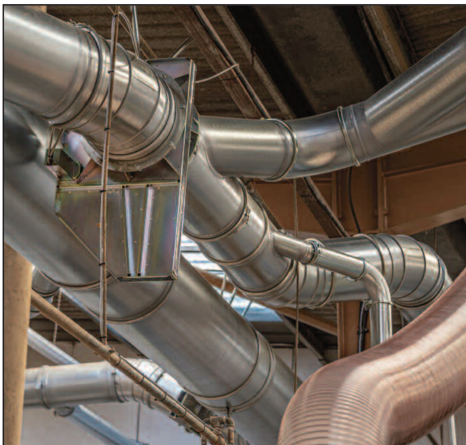
Ecogate's motorised dampers integrated into the Nordfab QF ductwork system automatically open and close as machines come on or offline.
