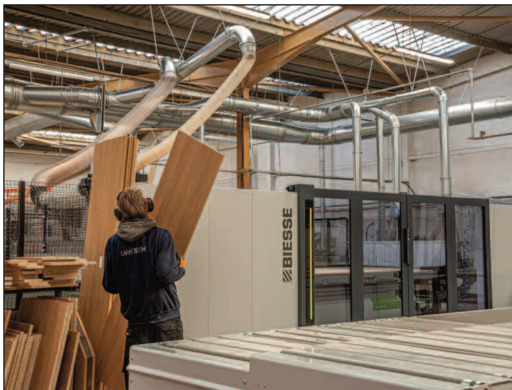
Installation of the new Biesse Rover B FT HD was the catalyst for upgrading the extraction system at Unitech Oxon Ltd.
