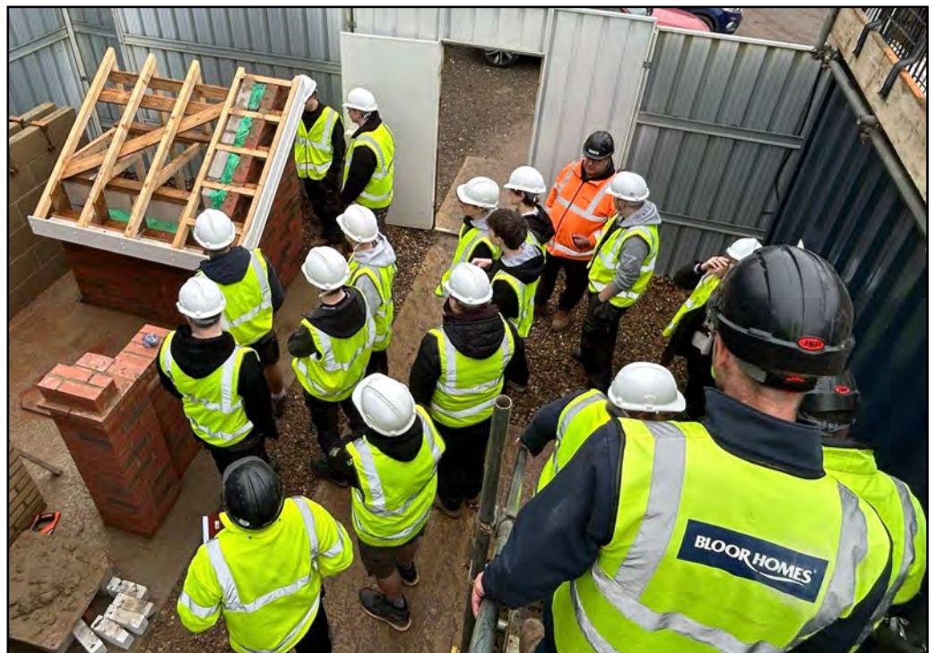
Carpentry students from the Eastern Education Group (part of West Suffolk College) had the opportunity to visit Bloor Homes at its live development at Thurston.
