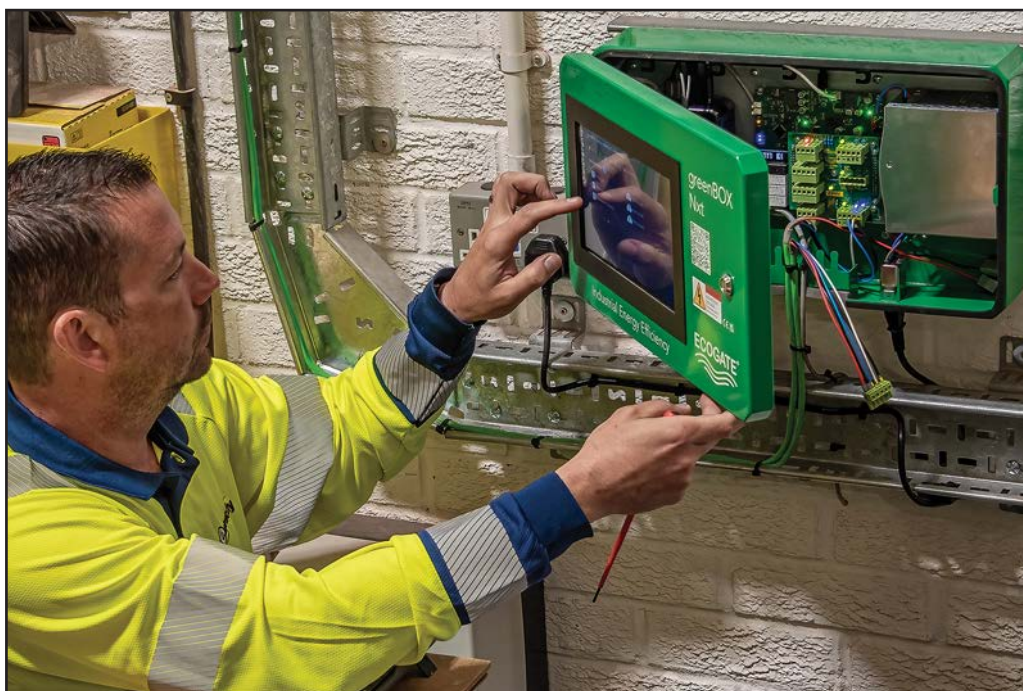
Installation and programming of the highly-intelligent greenBOX Nxt controller.
